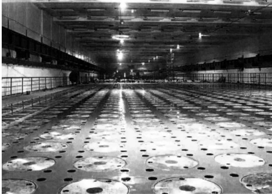
Figure 1. Interior picture of Mayak storage facility. A stack of containers, each holding two 2-kg plutonium-metal balls, can be stored under each square. 27
