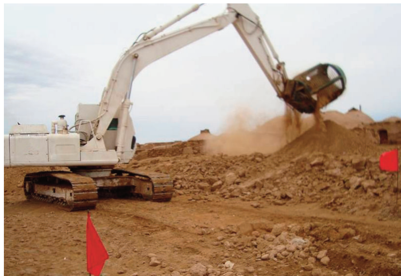
After Demining machine, in the same village, inspecting hazardous debris and, in the process, destroying physical borders between properties, which resulted in land disputes, due to the absence of owners and written land records.
