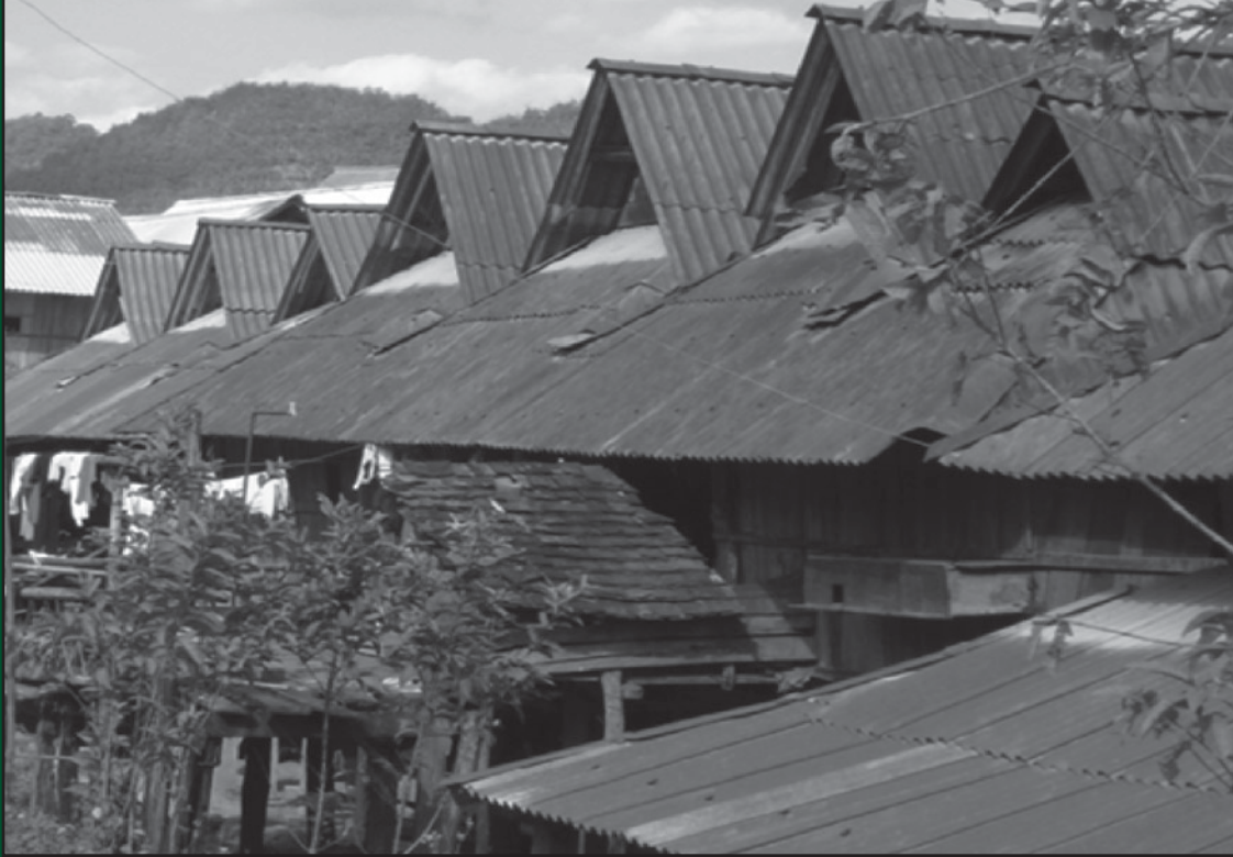
The use of asbestos as a roofing material is increasingly common in rural areas of Yunnan Province, posing health threats to both residents and the workers who produce the roofing materials. Photo Credit: YHDRA
