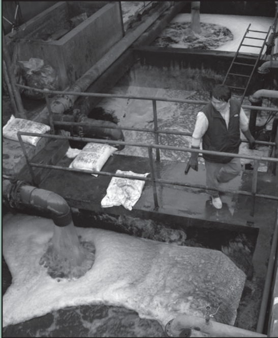
Aeration and biological treatment at a wastewater treatment plant in Guangdong Province. Photo Credit: Business for Social Responsibility
