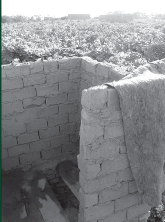
Outdoor Ecotoilet being built in Turpan by the Xinjiang Conservation Fund for eco-sanitation development in Xinjiang. Photo Credit: Daniela Salaverry
