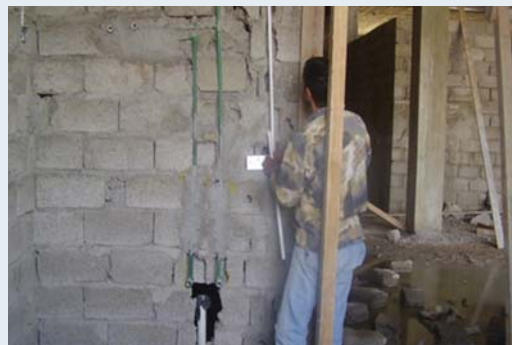
SIGIR inspects a poorly constructed block wall, one of many deficiencies that SIGIR identified at PHCs throughout the country.
