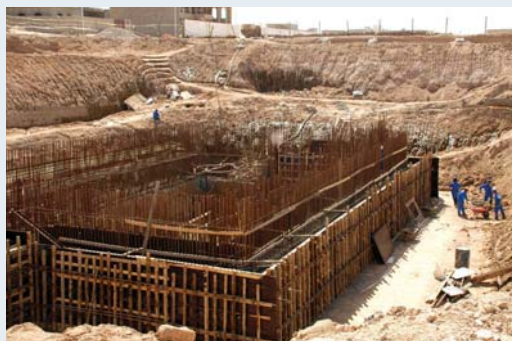
The Falluja Waste Water Treatment System project, on which the United States spent $100 million in U.S. funds, is not listed as a single project in the Iraq Reconstruction Management System. Instead, IRMS has 49 separate records, including records for project activities funded from the IRRF, CERP, and ESF. (U.S. Army photo)
