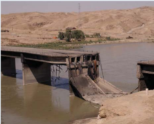
Coalition bombing damaged al-Fatah Bridge in 2003.
