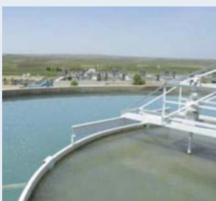
The Ifraz plant functioned at nearly 100% of capacity; 88% of the people serviced by the plant were satisfied with water availability; and 85% were satisfied with the water quality.
