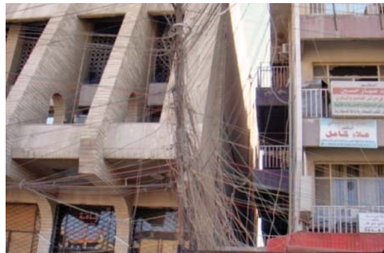
A tangle of consumer-installed electric wires carries power from private generators to households in central Baghdad. (Parsons Brinckerhoff photo)
