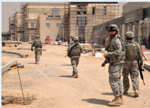
U.S. soldiers look over the grounds of the Basrah Children's Hospital under construction in May 2009. (U.S. Army photo)
