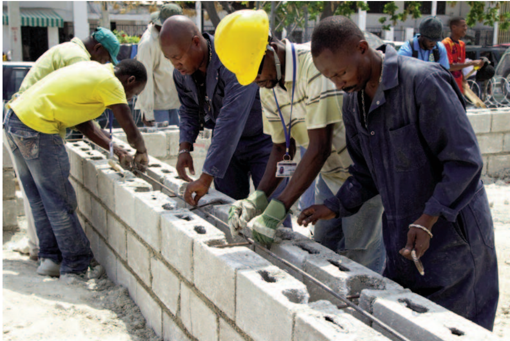
Following the destruction of the Haitian Parliament in the January 2010 earthquake, construction workers build a temporary Haitian Parliament facility with funds from MINUSTAH in March 2011. UN Photo/Logan Abassi.
