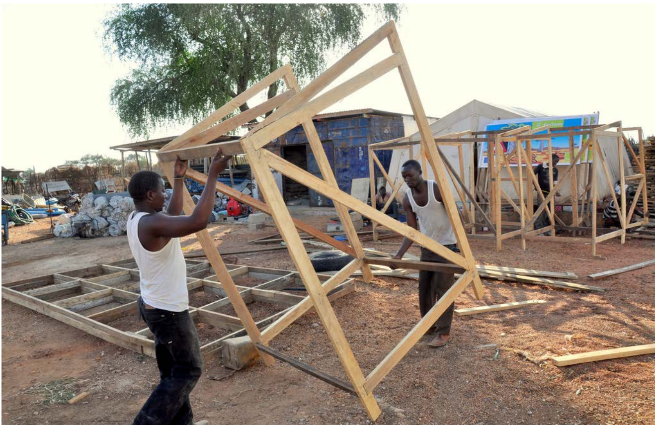
Oxfam workers constructing new latrines for families who have fled violence in conflict areas in Sudan.
