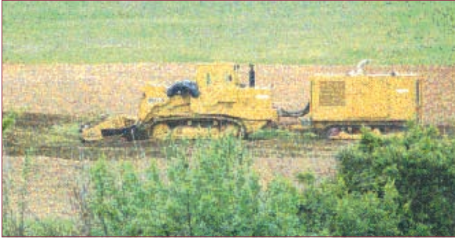
The Oracle system with the trailer-mounted power pack
