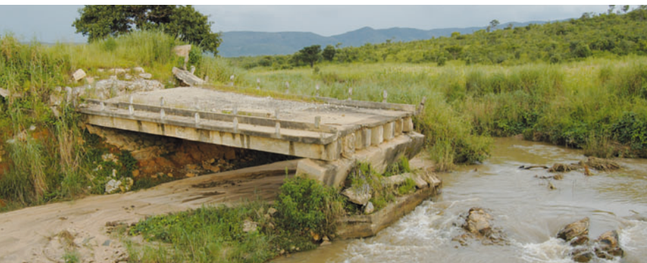
A bridge in need of reconstruction
